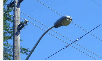
Faulty Street Lights
