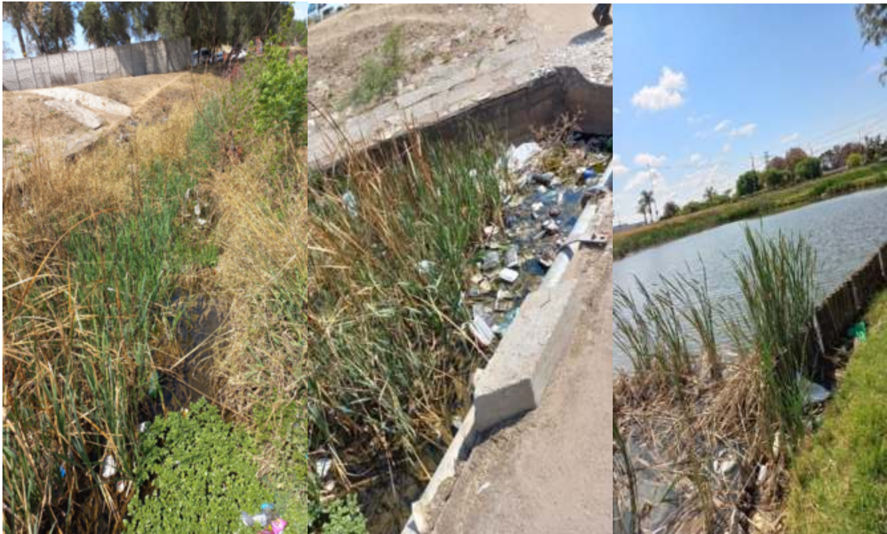
Diagram 183: Overgrown vegetation and litter noted in the drainage lines and stormwater infrastructure.
