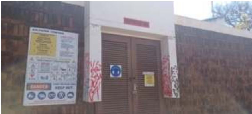
Diagram 177: Voortrekker Park substation to the east of the CBD
