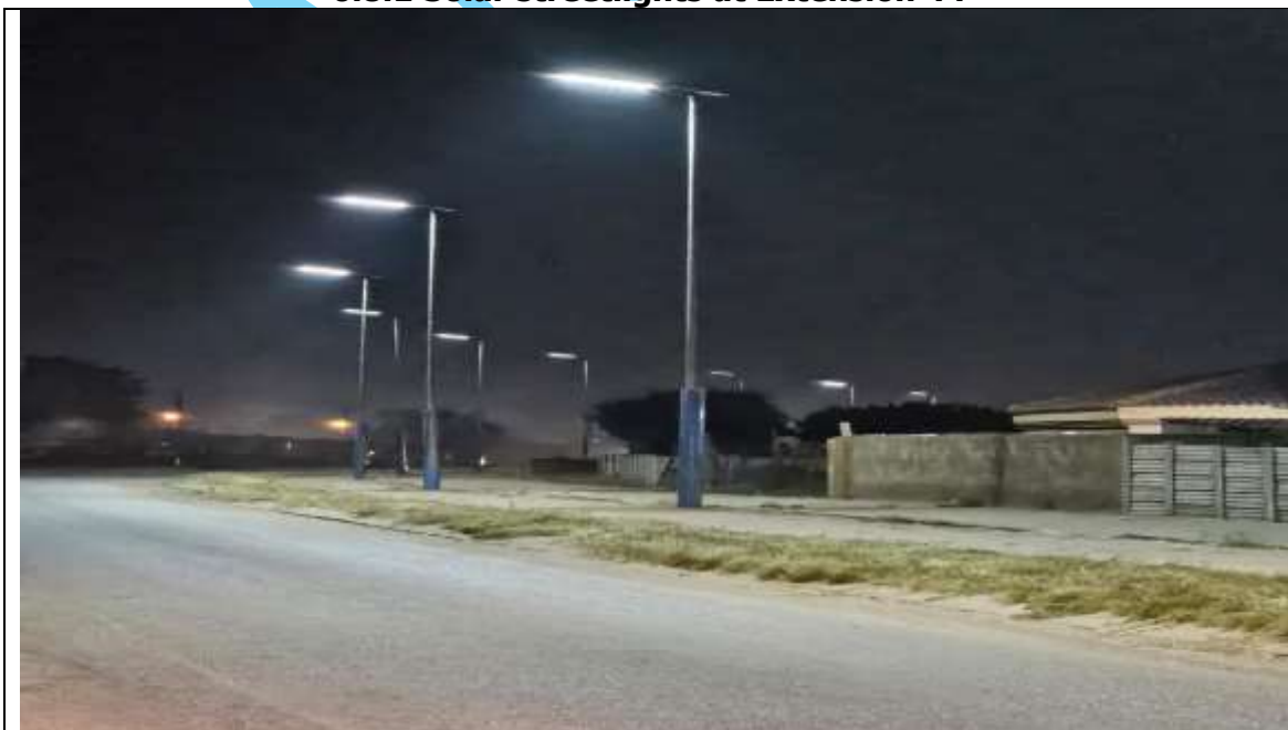
Solar streetlights at Extension 44
