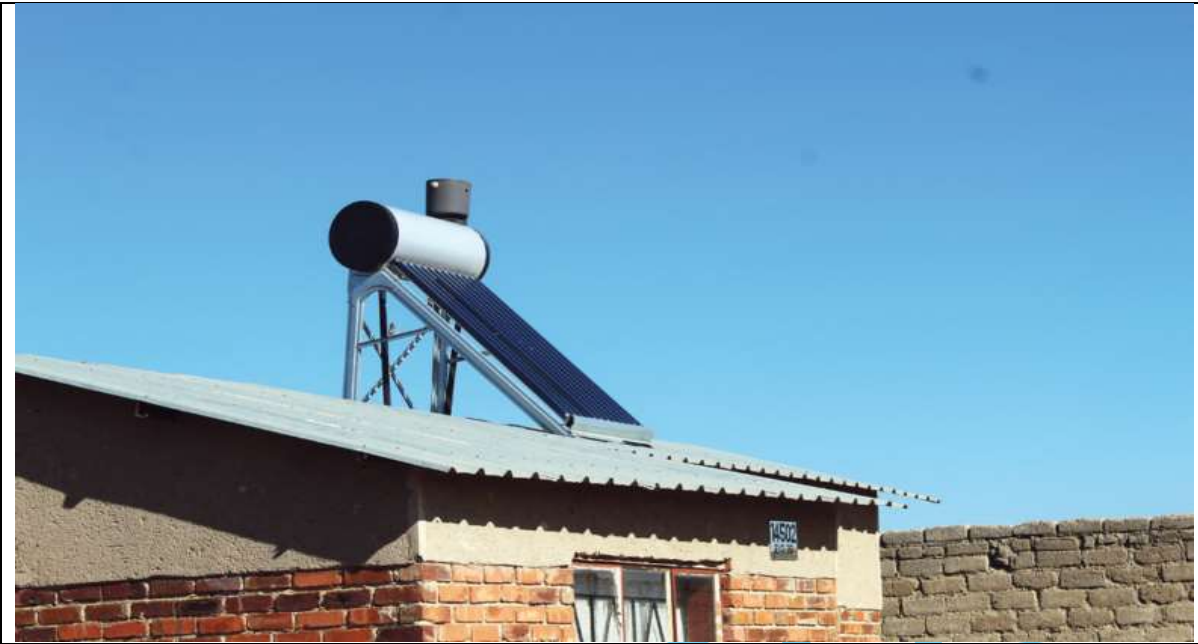
Solar geysers Installed at Seshego Ext 71 and 75 Source: PLK Energy Services Directorate
