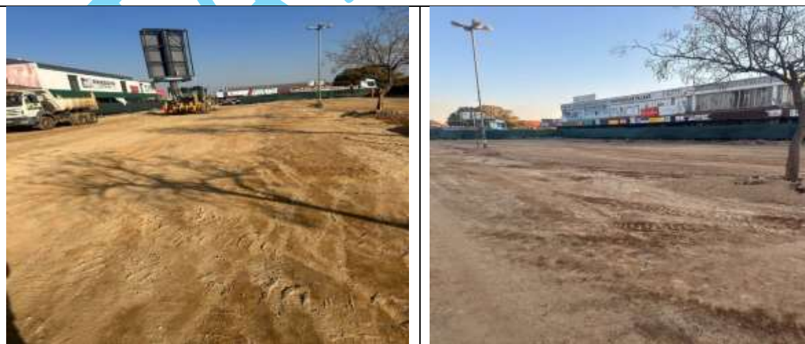
Upgrade of PT facilities at the Indian centre 1
