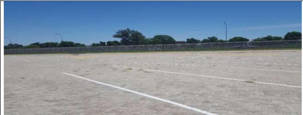
Leeto bus Daytime Layover Facility 1
