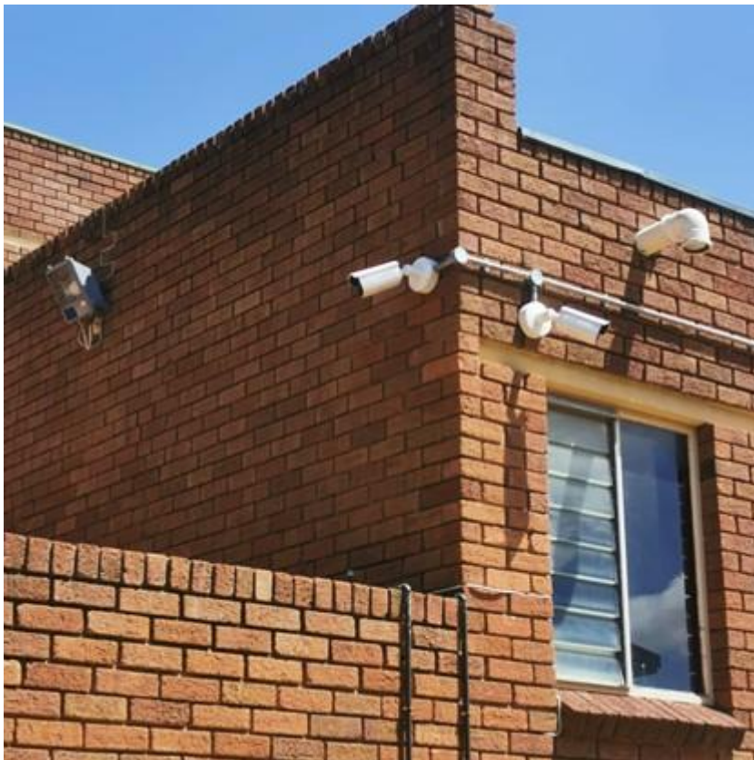
New installed cameras at Mankweng community hall
