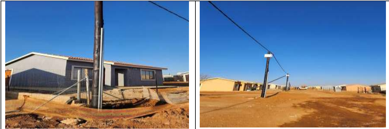
After Electrification Photos for Polokwane Ext 40
