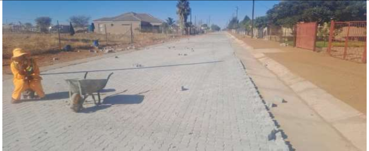
Paving of Street in Moletjie Ga Makibelo to Hlahla Ring Road (Ward 38)
