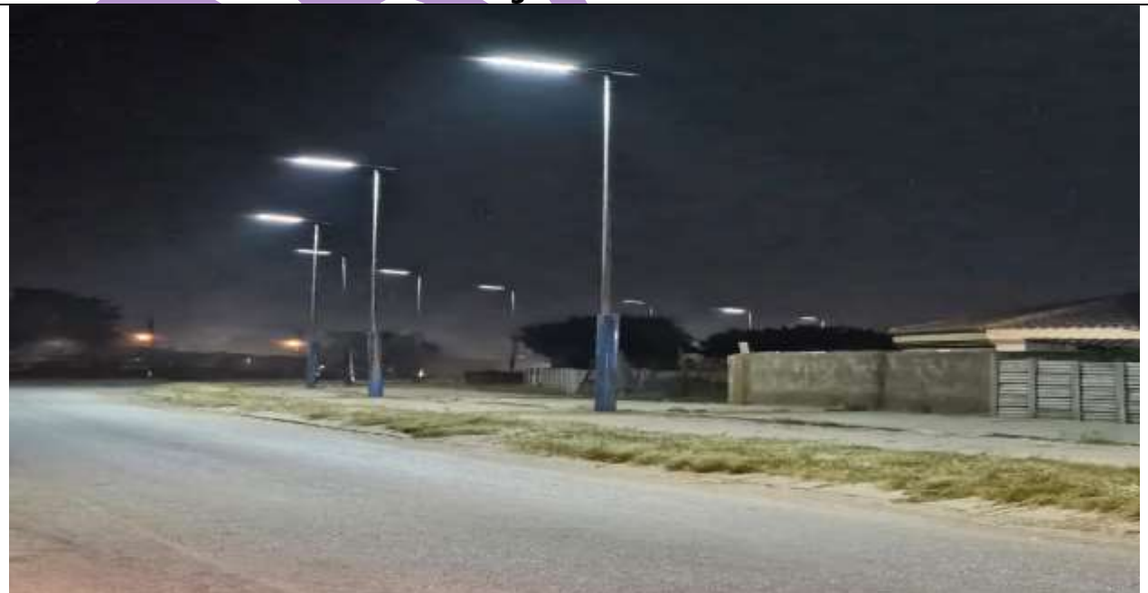
Solar streetlights at Extension 44
