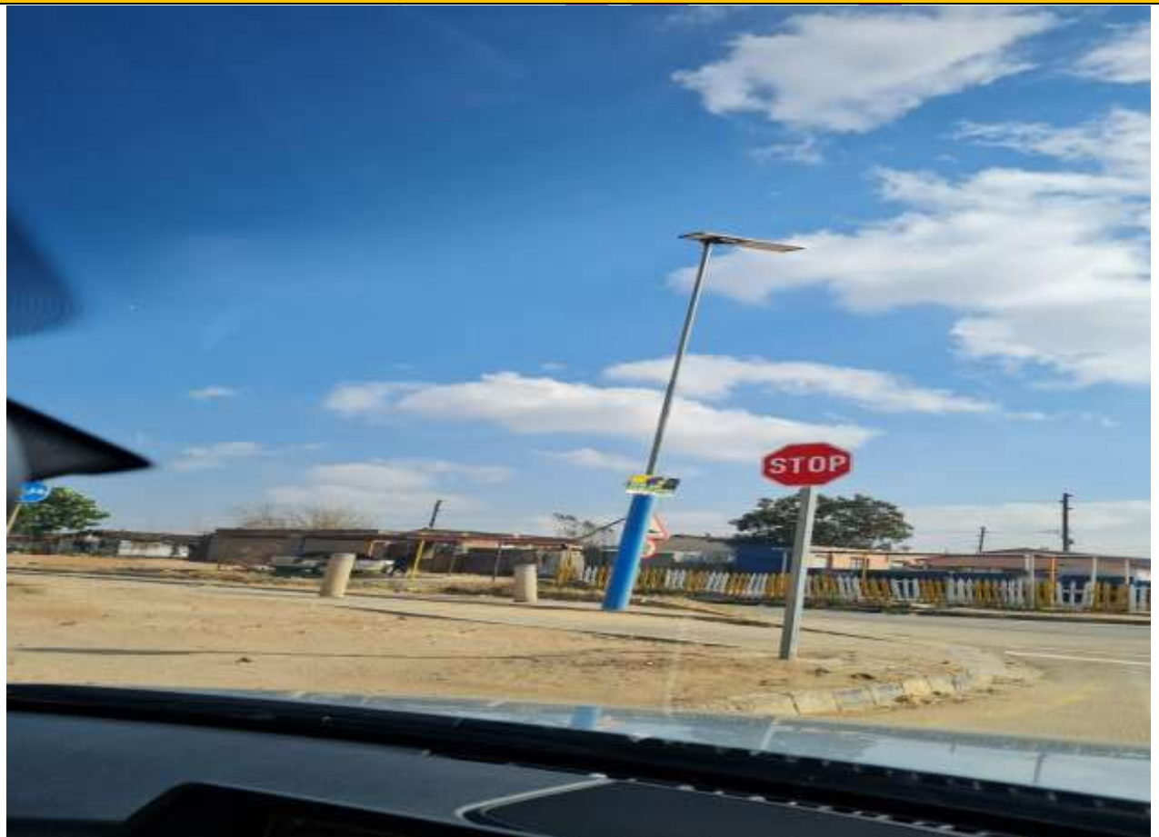
Solar streetlights at Extension 44
