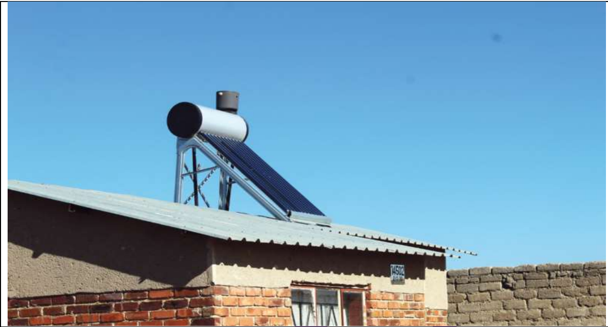
Solar geysers Installed at Seshego Ext 71 and 75 Source: PLK Energy Services Directorate
